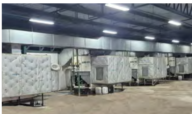
Optimisation of AHU temperature in control area
